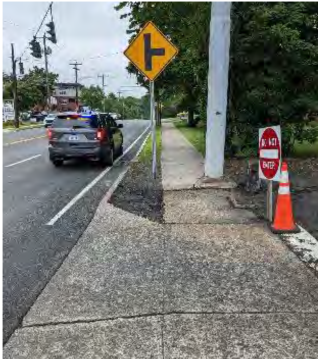
Exhibit 20: Damaged Sidewalk and Driveway Apron
