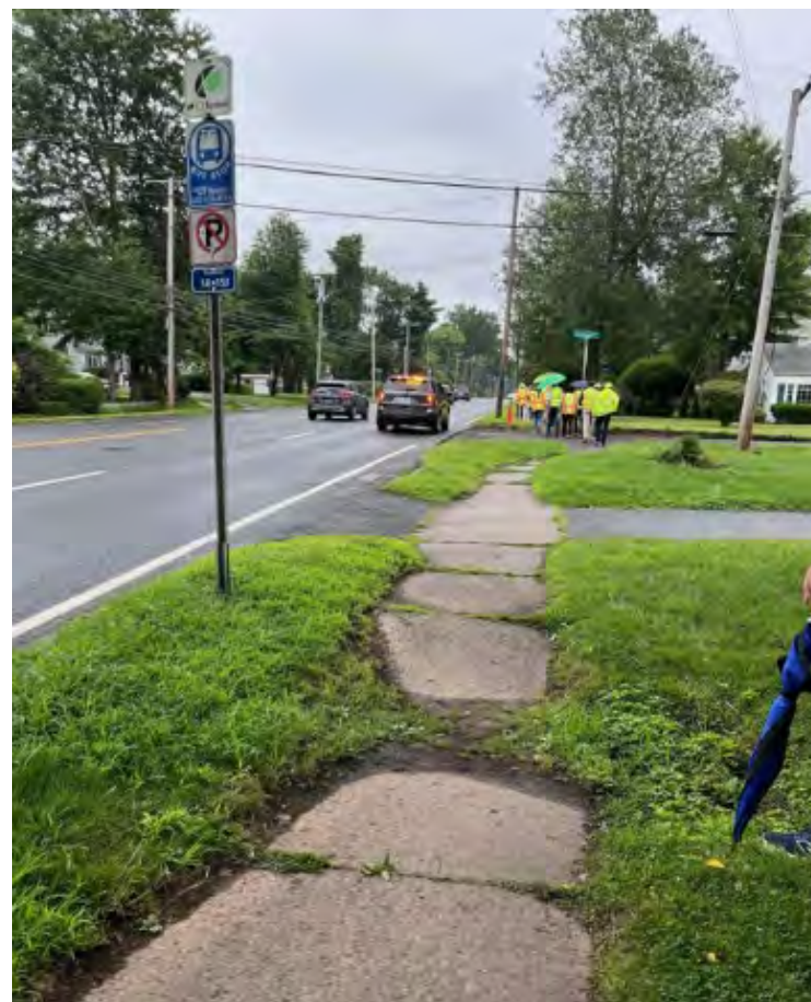
Exhibit 23: Sidewalk in Poor Condition Near Sherwood Drive
