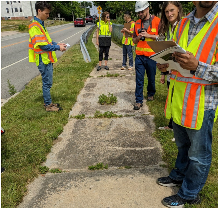
Exhibit 19: Sidewalk Condition on North Side of US Route 1
