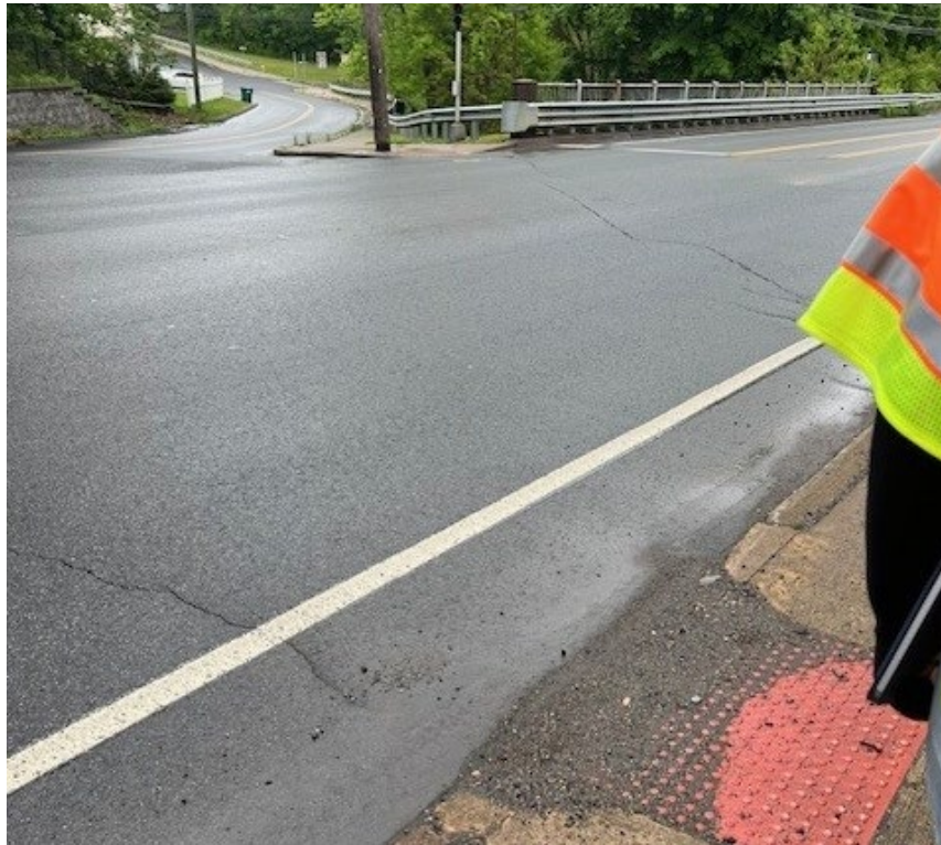
Exhibit 22: No Marked Crosswalks at Route 67 and Old Drive Intersection
