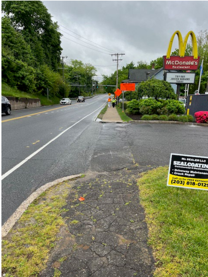
Exhibit 20: Damaged Sidewalk Near McDonald's Entrance
