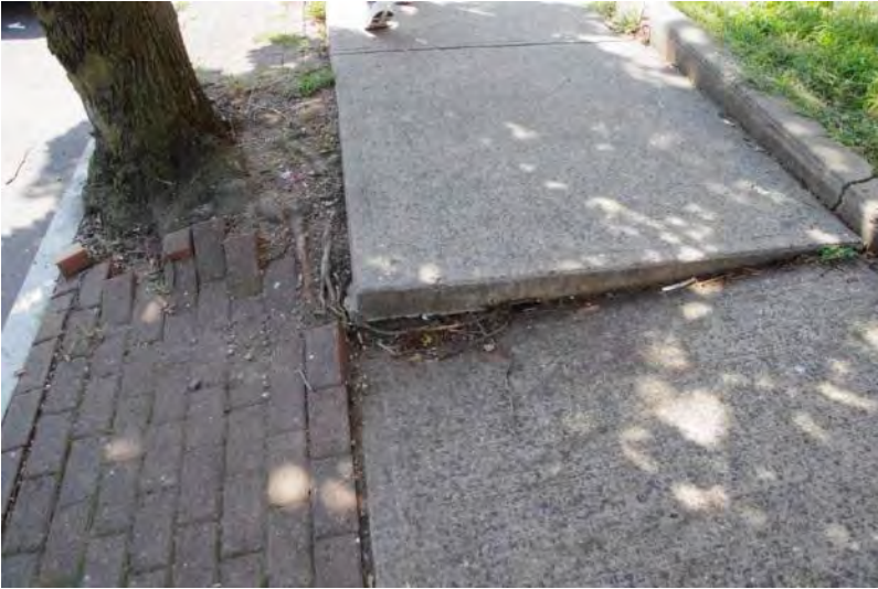
Exhibit 15: Sidewalk in Poor Condition along Route 127 (East Main Street)
