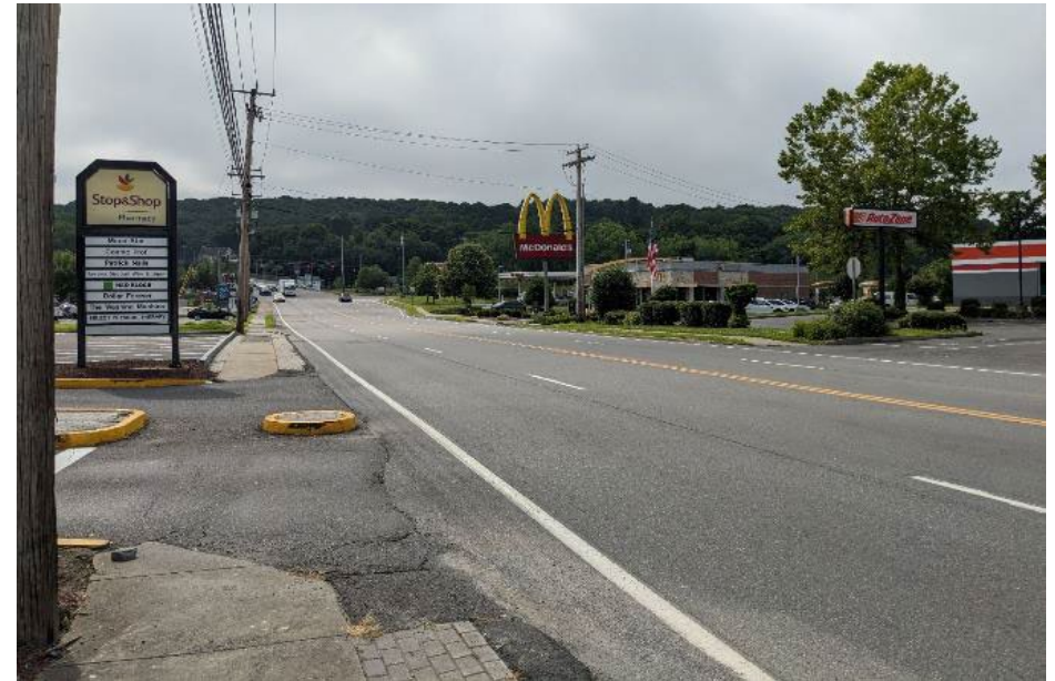
Exhibit 22: Pavers and Sidewalks in Poor Condition on Division Street
