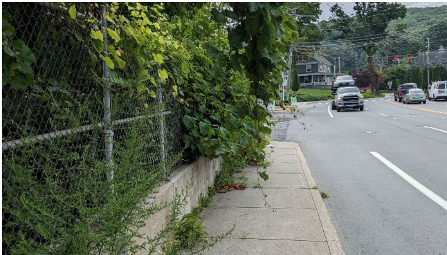
Exhibit 25: Overgrown Vegetation Along Bridge on Division Street Near South Division Street Underpass
