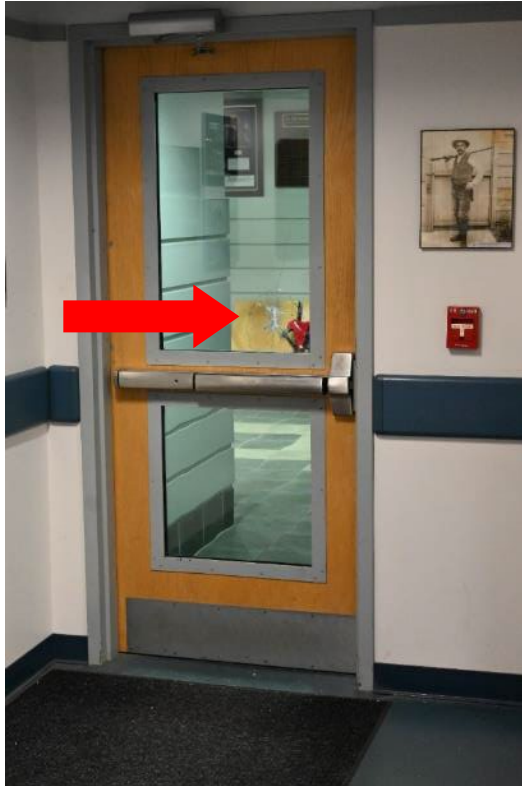
[North door with bullet strike from inside hallway]
