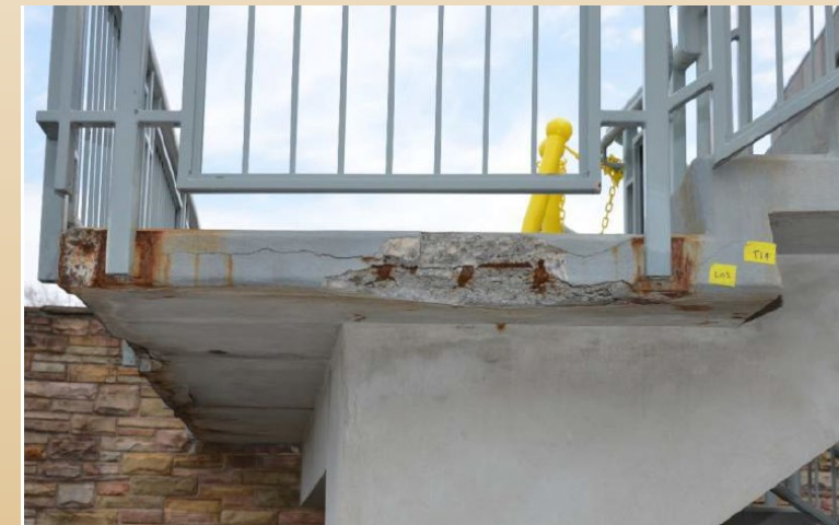
CRACKS AND RUST STAINS IN INTERMEDIATE LANDING
