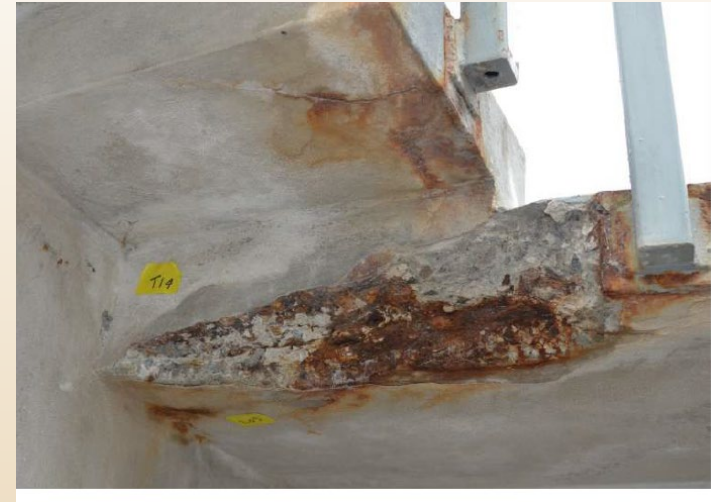
SPALL IN LANDING
