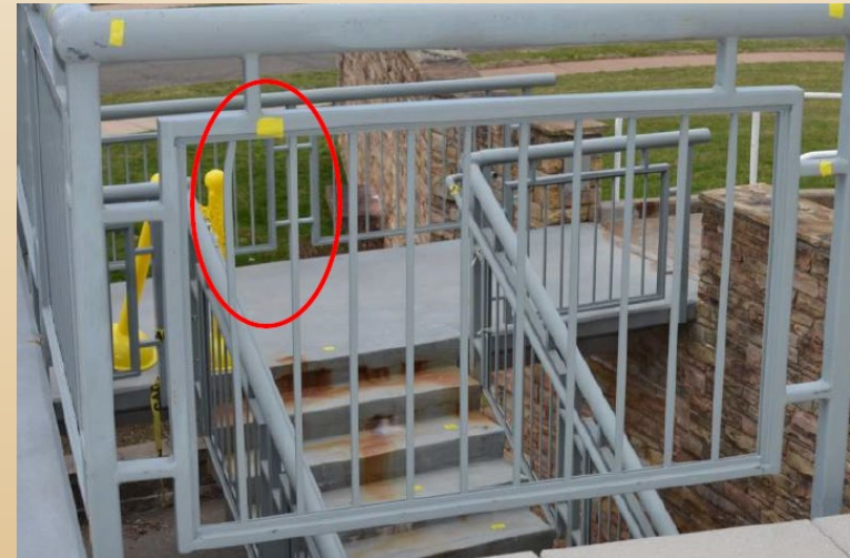
DAMAGED GUARD INFILL RAIL
