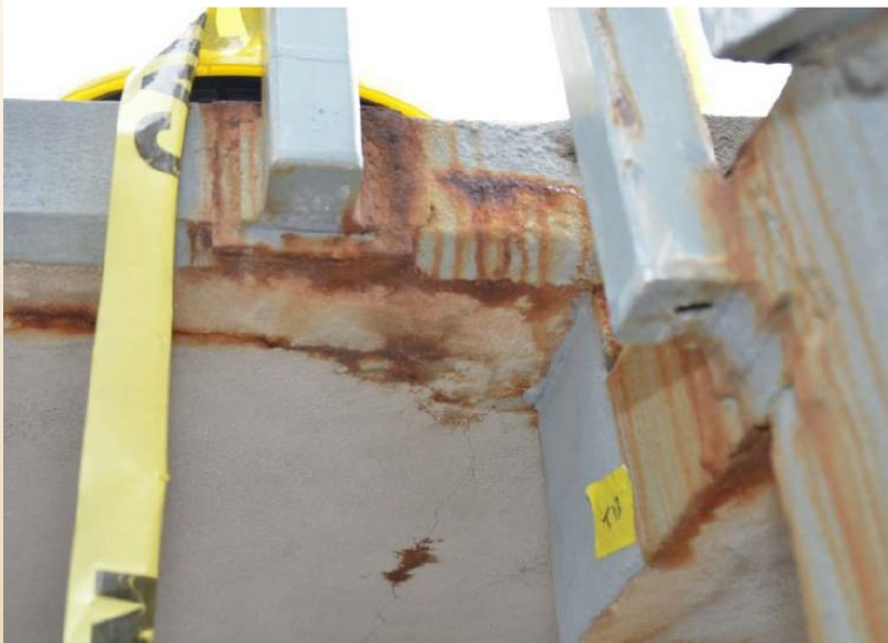
RUST STAIN AT GUARD POST CONNECTION
