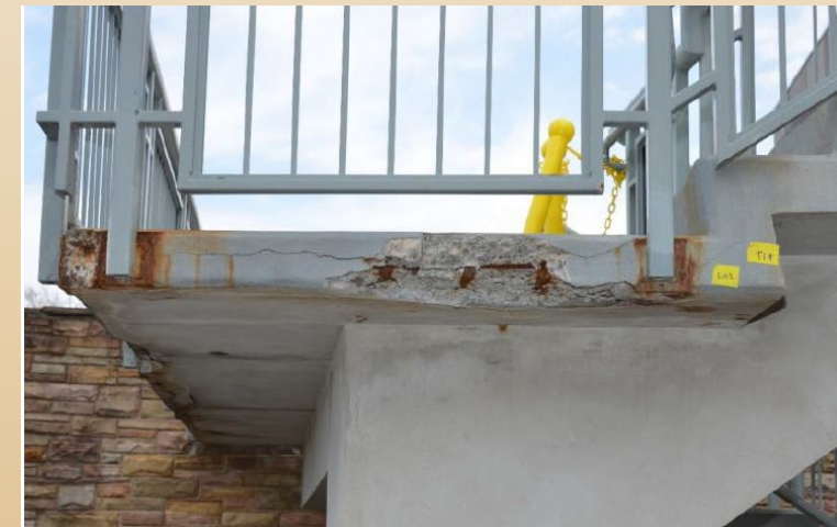
CRACKS AND RUST STAINS IN INTERMEDIATE LANDING
