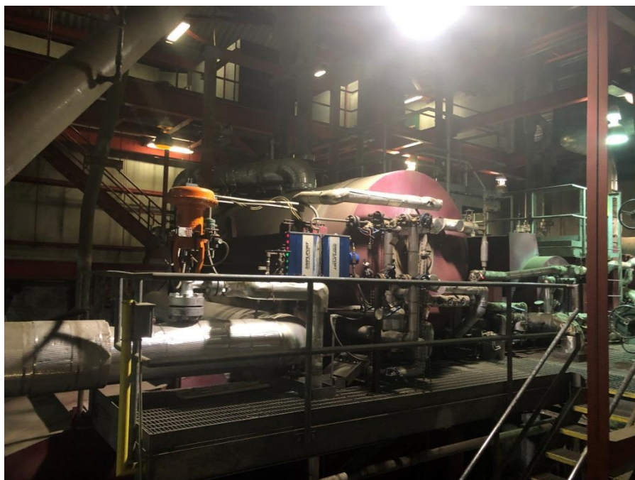
G.E. Steam Turbine
