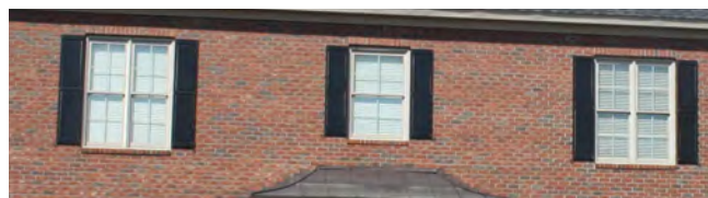
Inappropriately Scaled Shutters.
