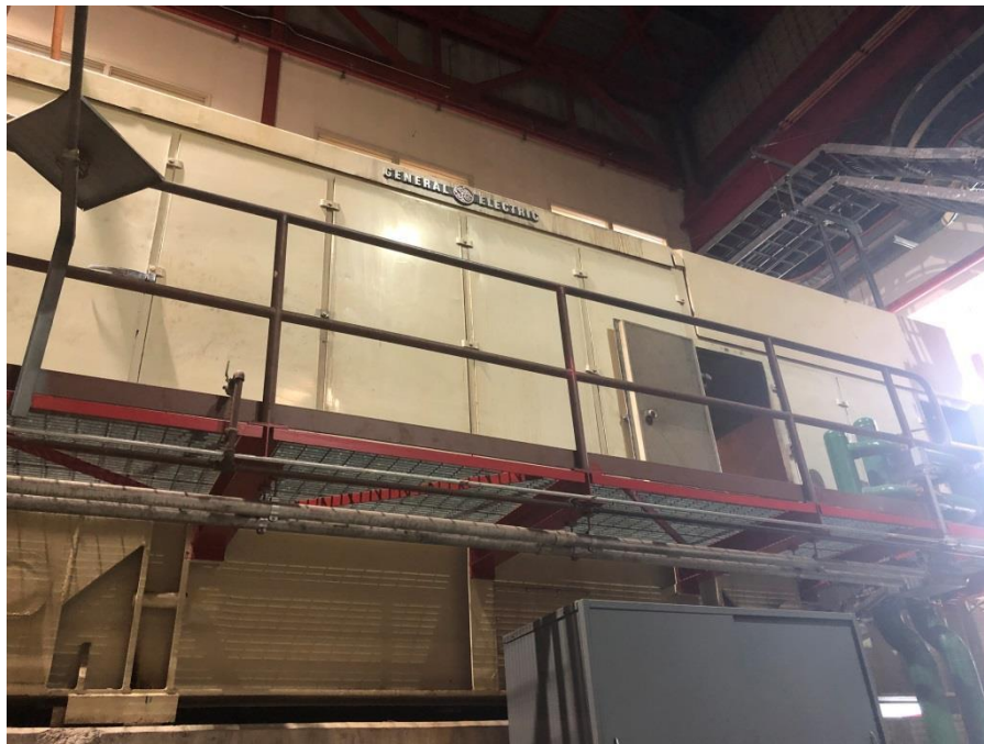
G.E. Frame 6 Gas Turbine
